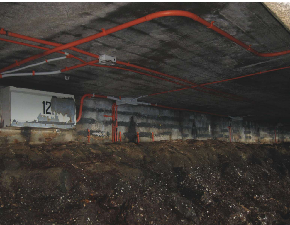
A control unit installed underneath the wharf was part of the original ICCP system. Photo courtesy of Atef Cheaitani.
