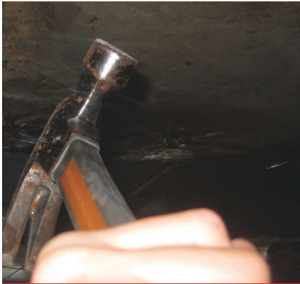
It took a crew of six people, accessing the structure by boat and land, about two weeks to hammer test the entire concrete surface underneath the wharf. Photo courtesy of Atef Cheaitani.
