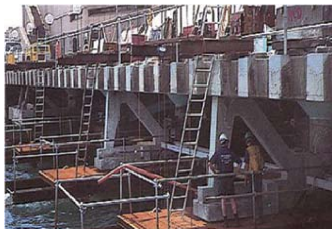
Figure 2: Cathodic Prevention applied to the Western Underbroadwalk of the Sydney Opera House in 1995-96 (First cathodic prevention system in Australia)
