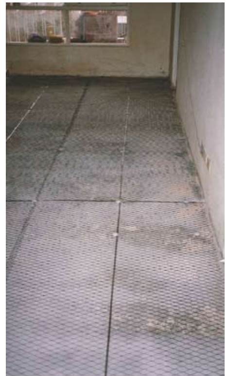
Figure 1: MMO Titanium mesh anode applied to the slab of a unit in Mosman, Sydney in 1989
